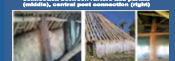
Interlocking connection (left), lashed connection between rafters and purlins (middle), central post connection (right)
